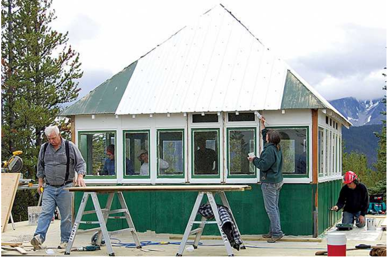
Volunteers from the Houston community help with the restoration work on Owen Hills Lookout
